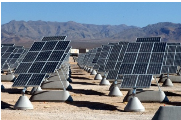
Figure 4. Layla solar power station [6]
