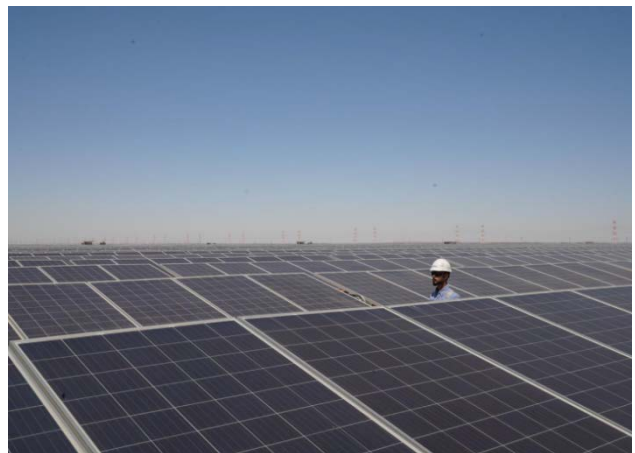
Figure 5. Sakaka power plant [7]
